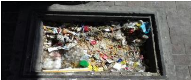
Vandalized hydrants and dumping in chambers
